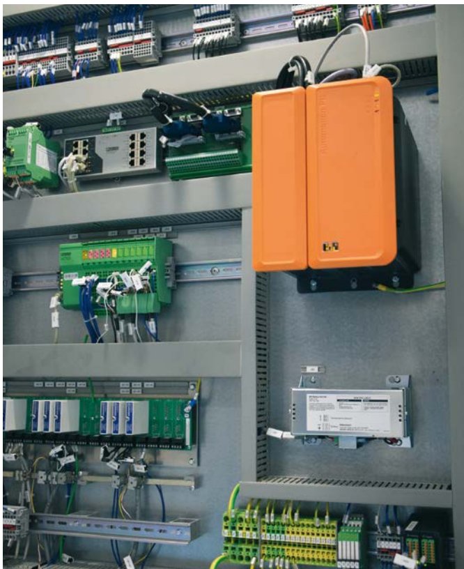
On the operational level, these PCs run SCADA systems and the SQL database, while on the machine level they are used to carry out function tests.
