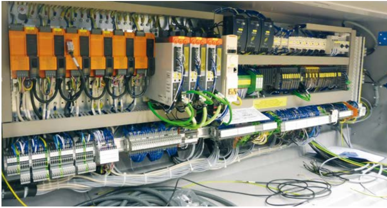
To ensure its ability to accommodate customer requests, Müller Martini builds all of its control panels in house.
