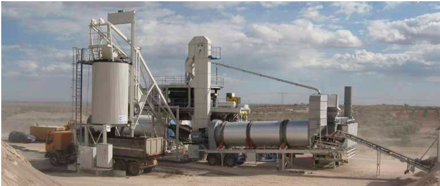
The mobile mixing plant with a silo that holds up to 30 tons of material and can be loaded directly from a truck.
