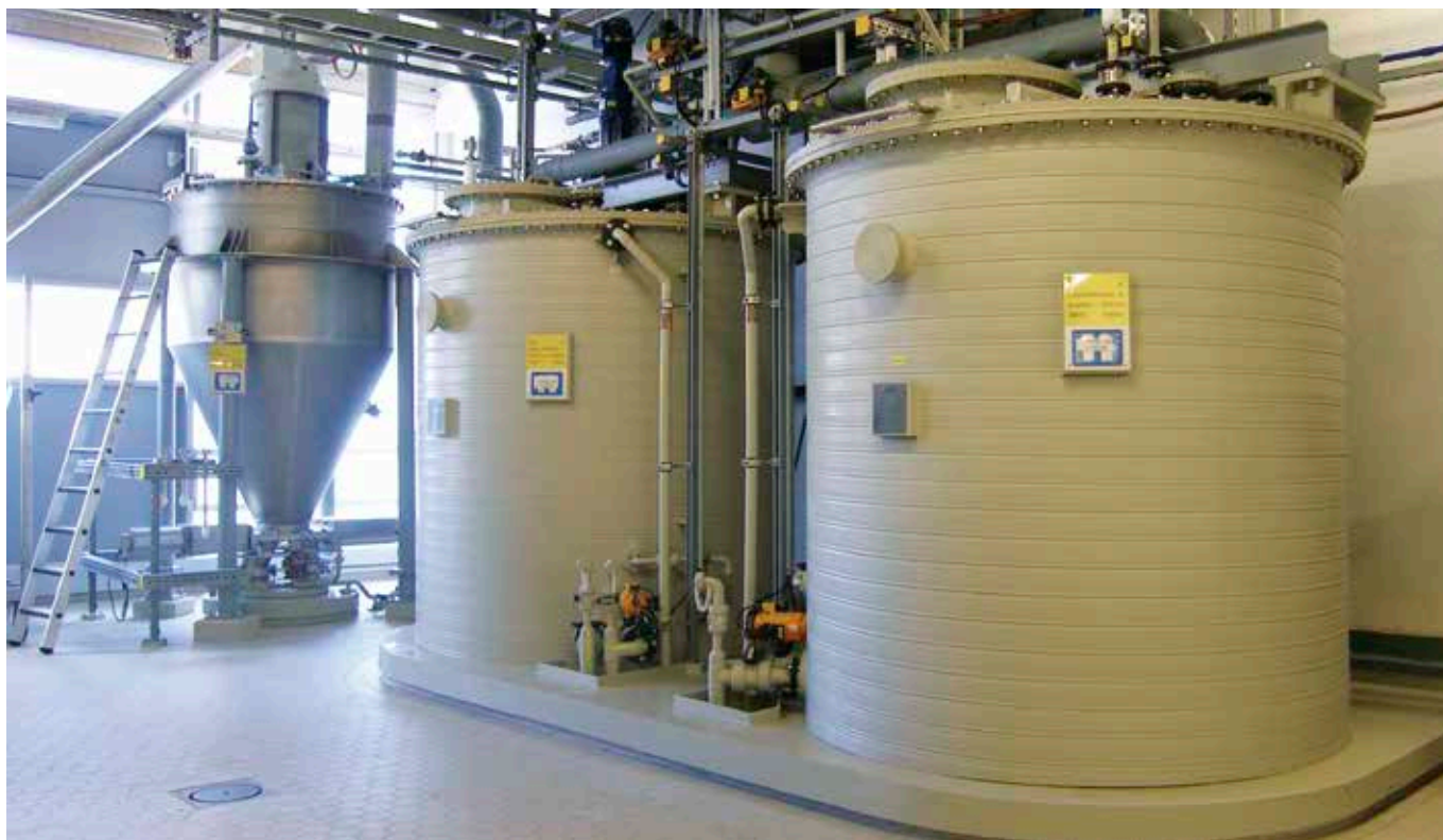
At Merck's state-of-the-art production plant for inorganic salts, every stage in the process – including crystallization – is controlled by the fully automated APROL process control system.
